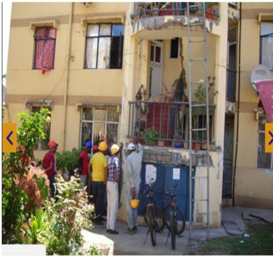
Beau Vallon Housing Estate before rehabilitation
